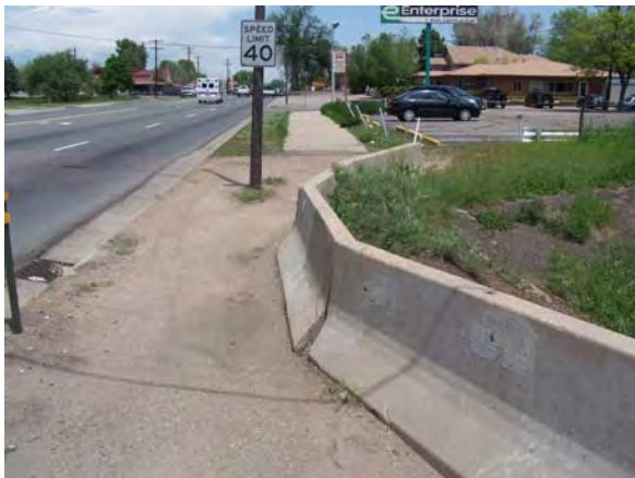
EXHIBIT 1-4: MISSING SIDEWALK SEGMENT SOUTH OF 12TH AVENUE
