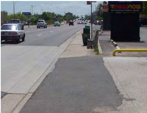
EXHIBIT 1-3: MISSING SIDEWALKS AND OBSTRUCTIONS NEAR 5TH AVENUE
